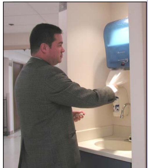
With a wave of the hand, new proximity-sensing towel dispensers produce a clean paper towel after handwashing. “Every time you can eliminate the need for people to touch things, you reduce opportunities to transmit infection,” says Environmental Services Director, John Merkt. Looking for more such opportunities, Merkt recently had sensor-activated lights installed in supply rooms.
